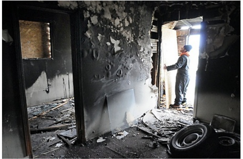
Neighborhood volunteers Harrison Roberts and his wife Erica work on boarding up.
