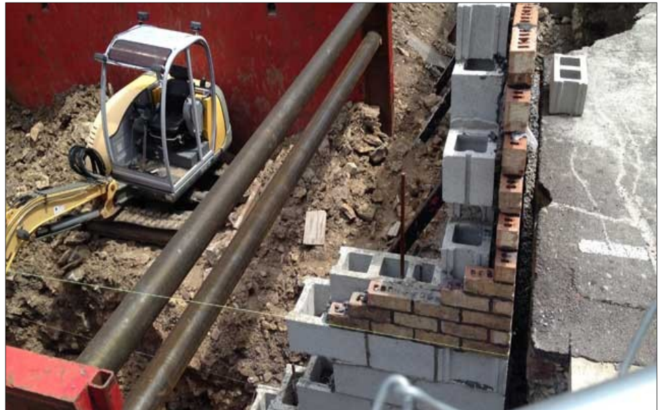
Above: Equipment sits unused in a deep hole next to Demonbreun where a former building stood. Owners hoped to have The Diner open by Spring, which now hinges on committee decisions.
