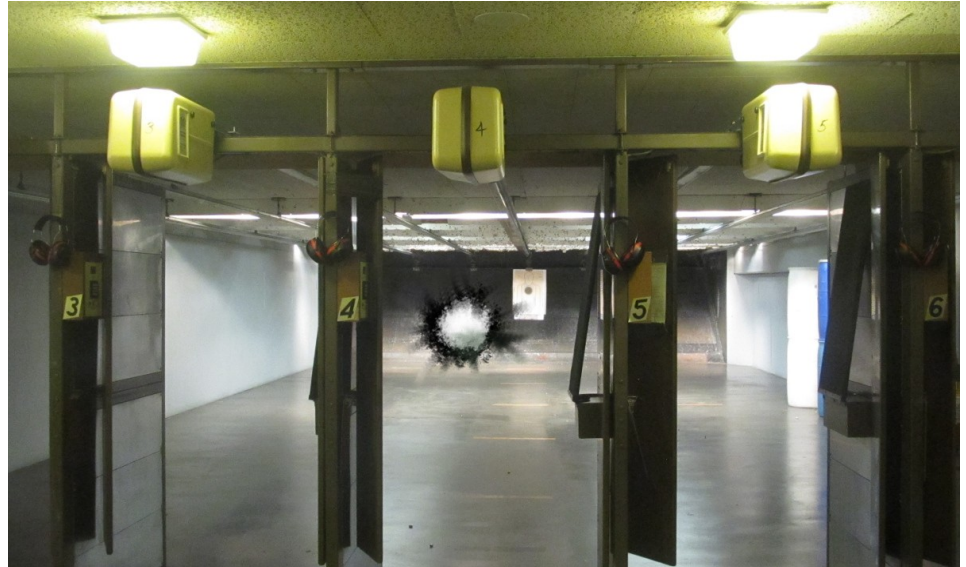
Attracting the attention of Federal law enforcement, a large hole was blown out of the back of a firing range off of Nolensville Road.
